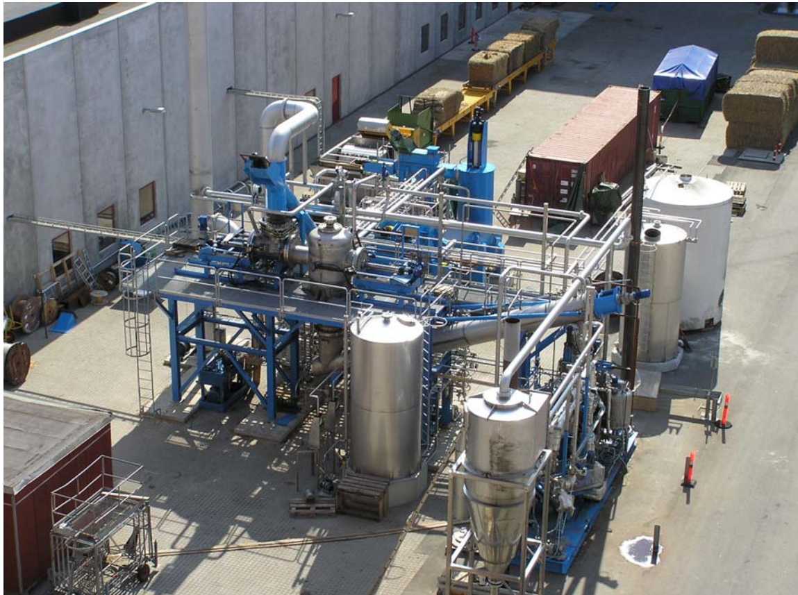
Figure 2 Pilot plant 1000 kg/h (straw reception, mechanical treatment and thermal pretreatment)
